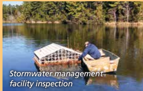
Overgrown and damaged outflow
